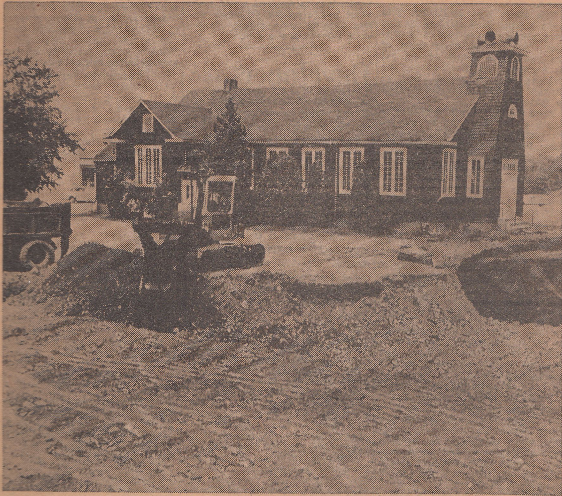
Excavation for the new Ponds Reformed Church at the corner of Oak Street and Ramapo Valley Road in Oakland gets under way this week. Photo was taken yesterday afternoon. Construction is due to begin as soon as excavation is completed.
